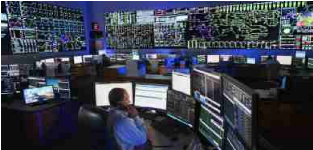
▲ PJM Control Room ( https://insidelines.pjm.com )
